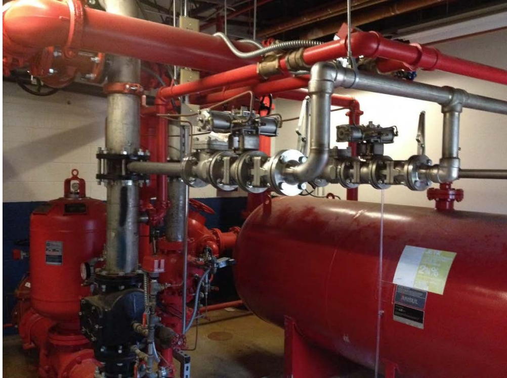
Photo 1: View of Hanger 1 HEF MEC Room.
