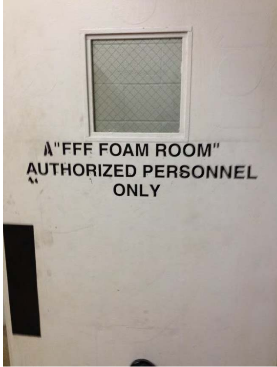
Photo 3: View of interior door to MEC room of West Fuel Cell.
