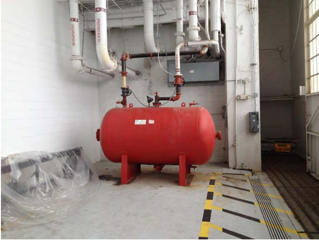
Photo 3: View of Hangar 10 AFFF tank and trench drain.
