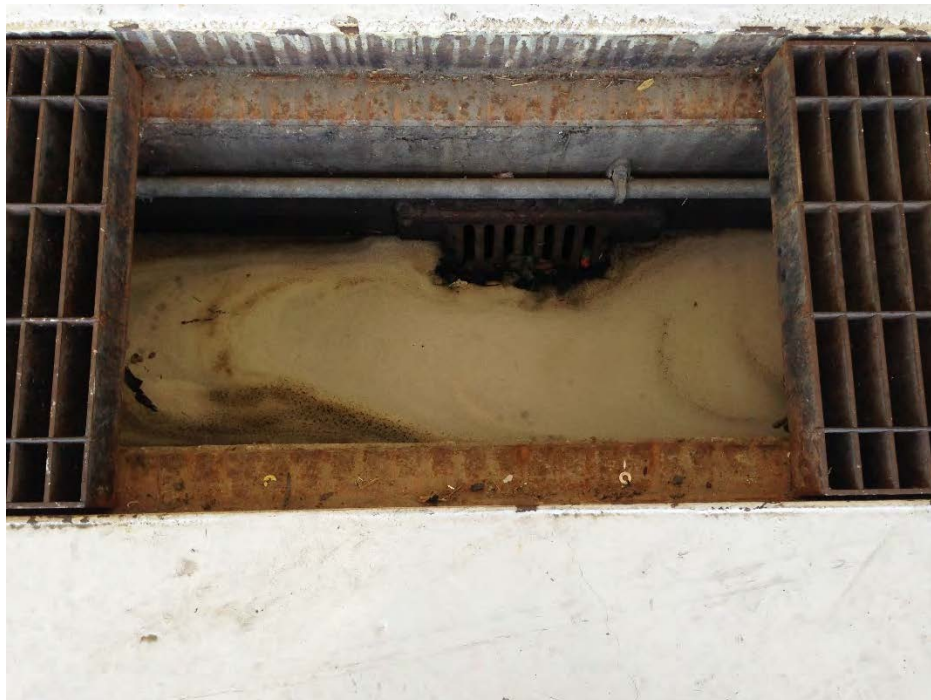
JBA provided photo of 29 July 2013 AFFF release at building 3629 in Trench drain
