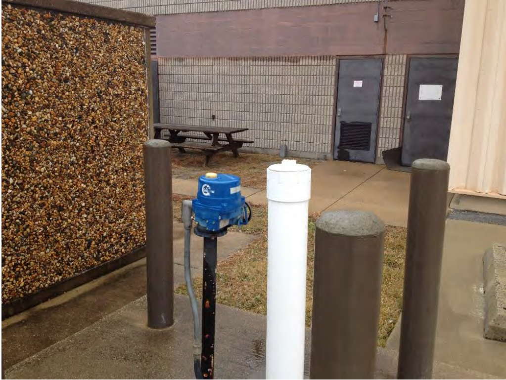
Photo 1: View of southwest corner of Hangar 18. Isolation valve and containment are with MEC room in background.
