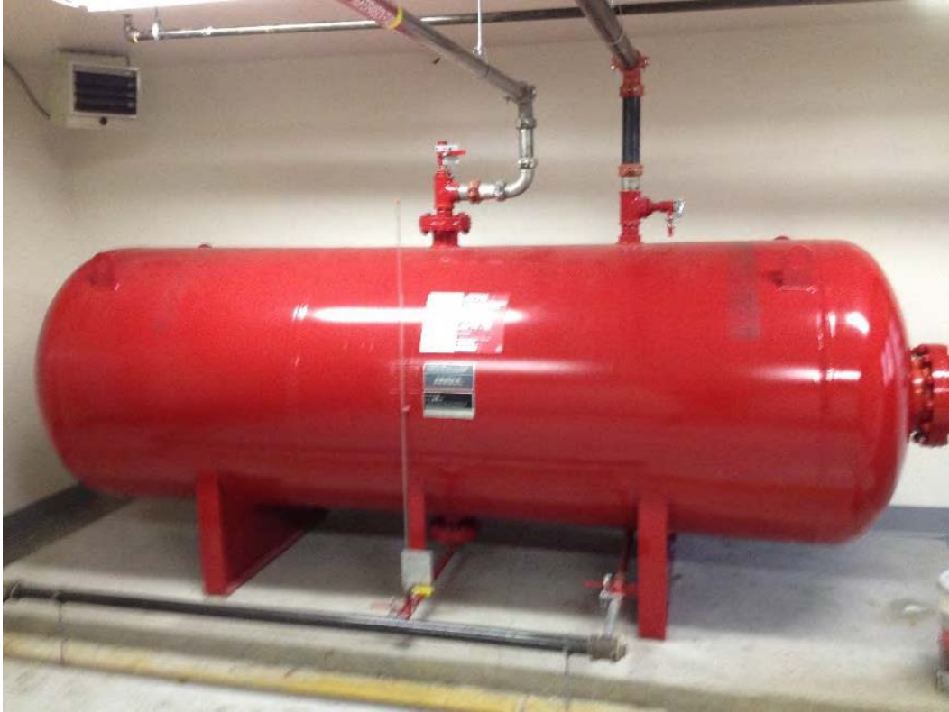
Photo 1: View of Hangar 7 MEC room - HEF.
