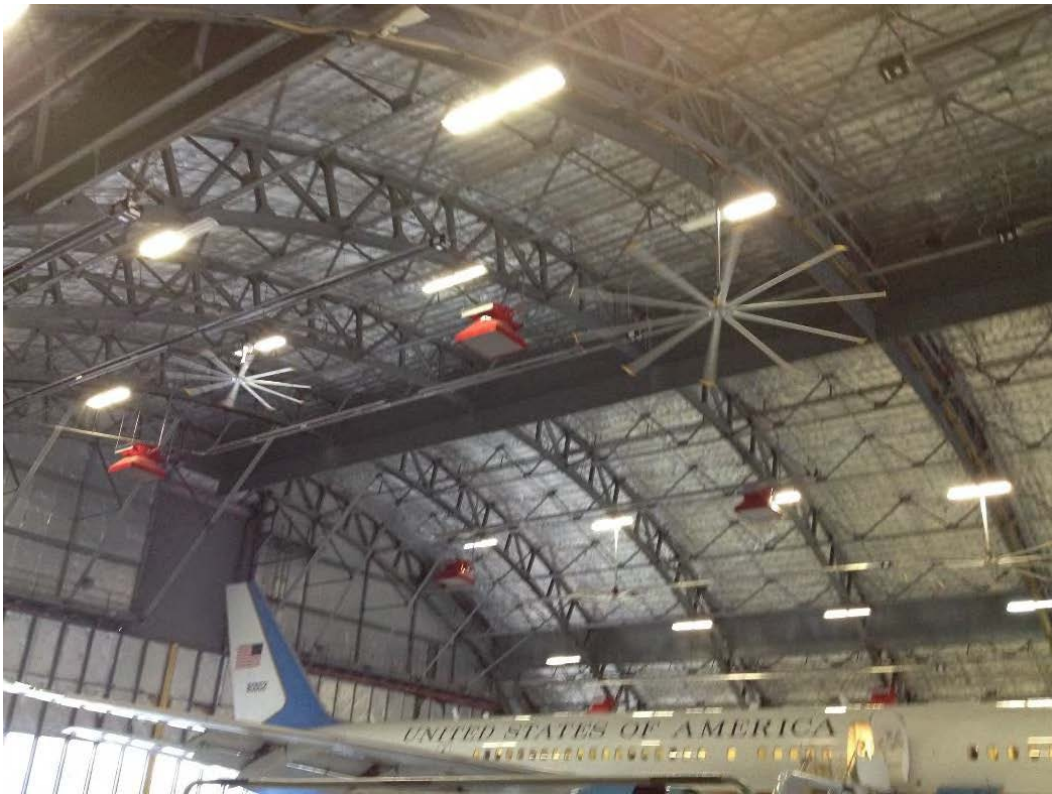
Photo 2: View of fire suppression system in Hangar 7.
