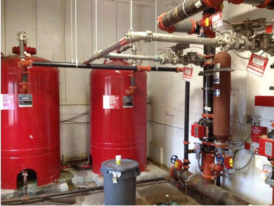
Photo 1: View of Hangar 4 MEC room.
