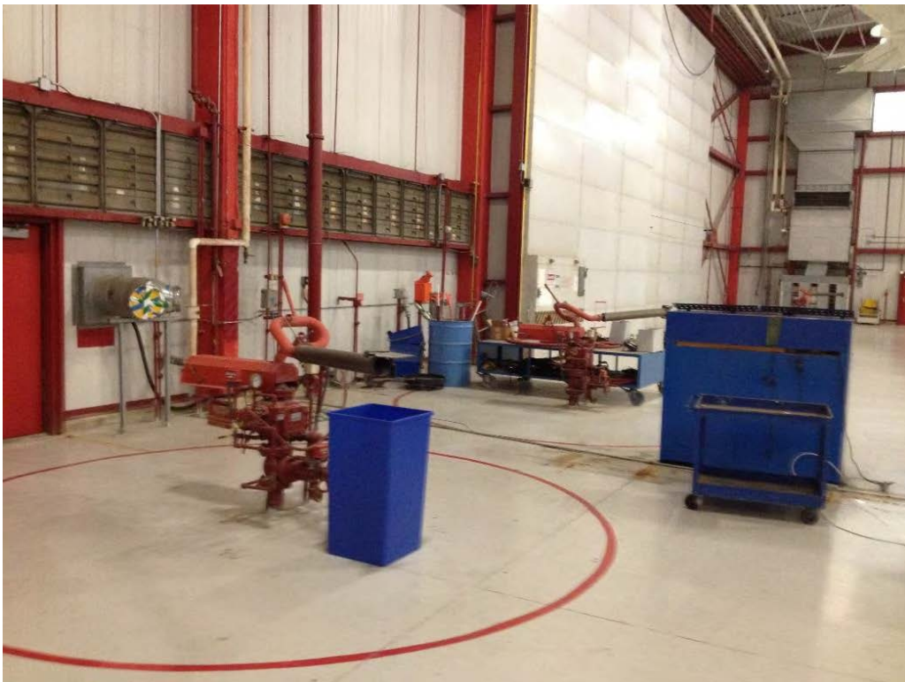
Photo 2: View of Hangar 18. AFFF floor cannon.
