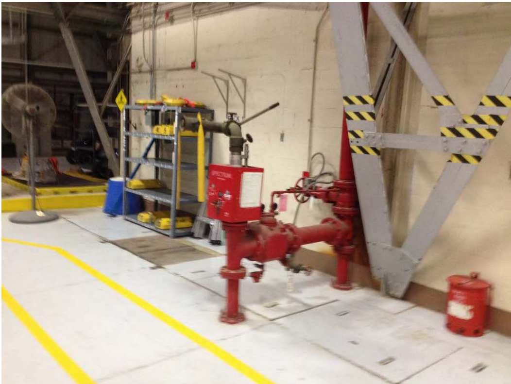
Photo 2: View of Hangar 8 AFFF foam cannon.
