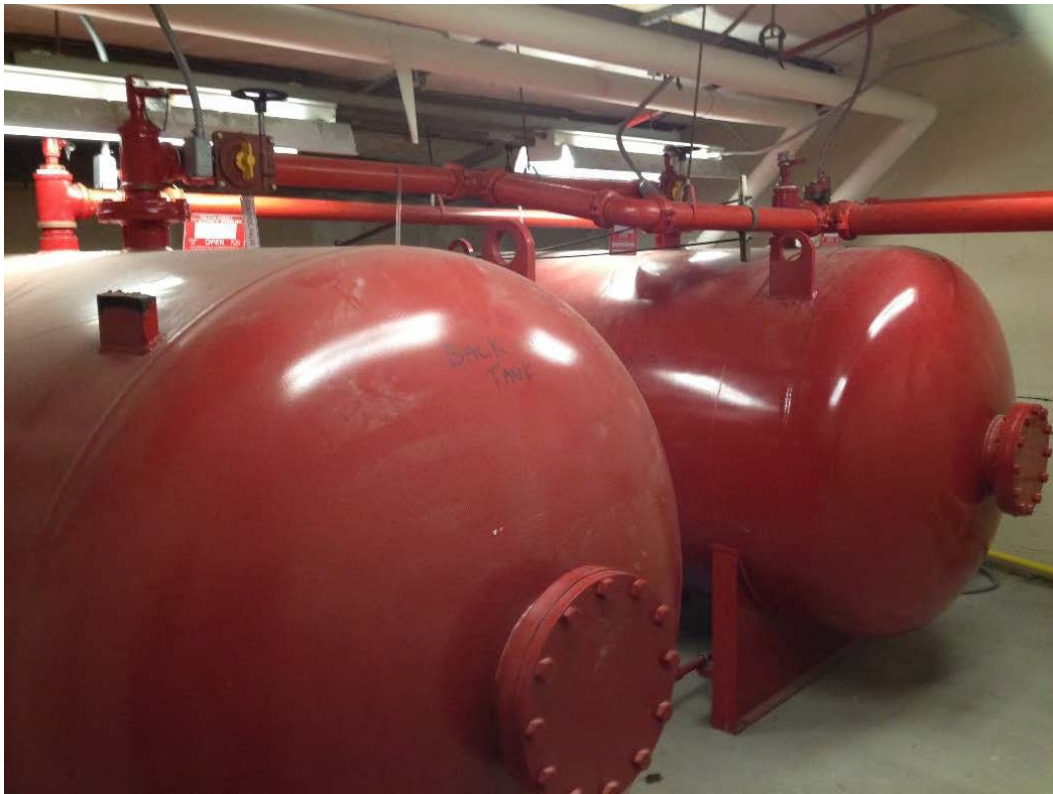
Photo 2: View of Hangar 9 MEC room with twin 1,100 gallon AFFF tanks.
