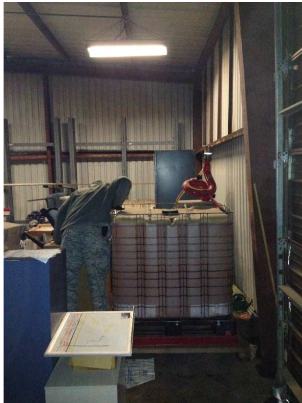
Photo 2: View of BLDG 3444 interior with AFFF 250 gallon foam cannon.
