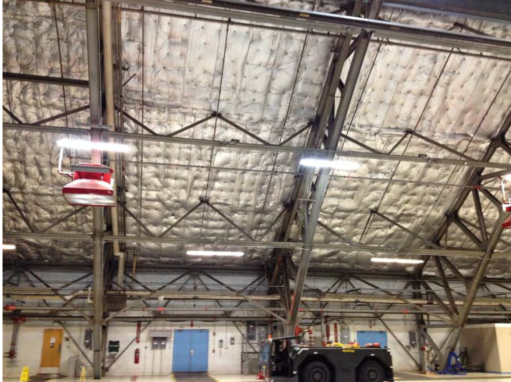
Photo 1: View of Fire Suppression system in Hangar 3.
