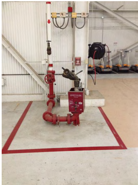
Photo 2: View of Hangar 11 AFFF foam cannon.
