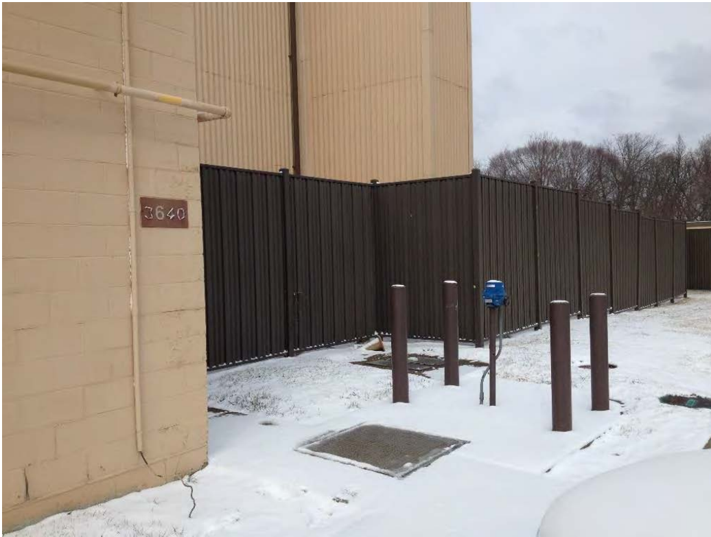
Photo 4: View of Hangar 10 exterior AFFF secondary containment located on east side of Hangar.
