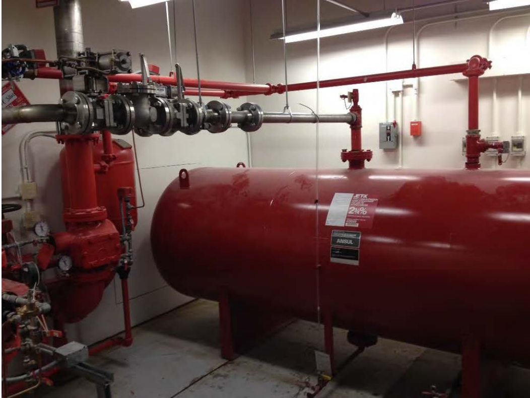
Photo 1: View of Hangar 6 MEC room.
