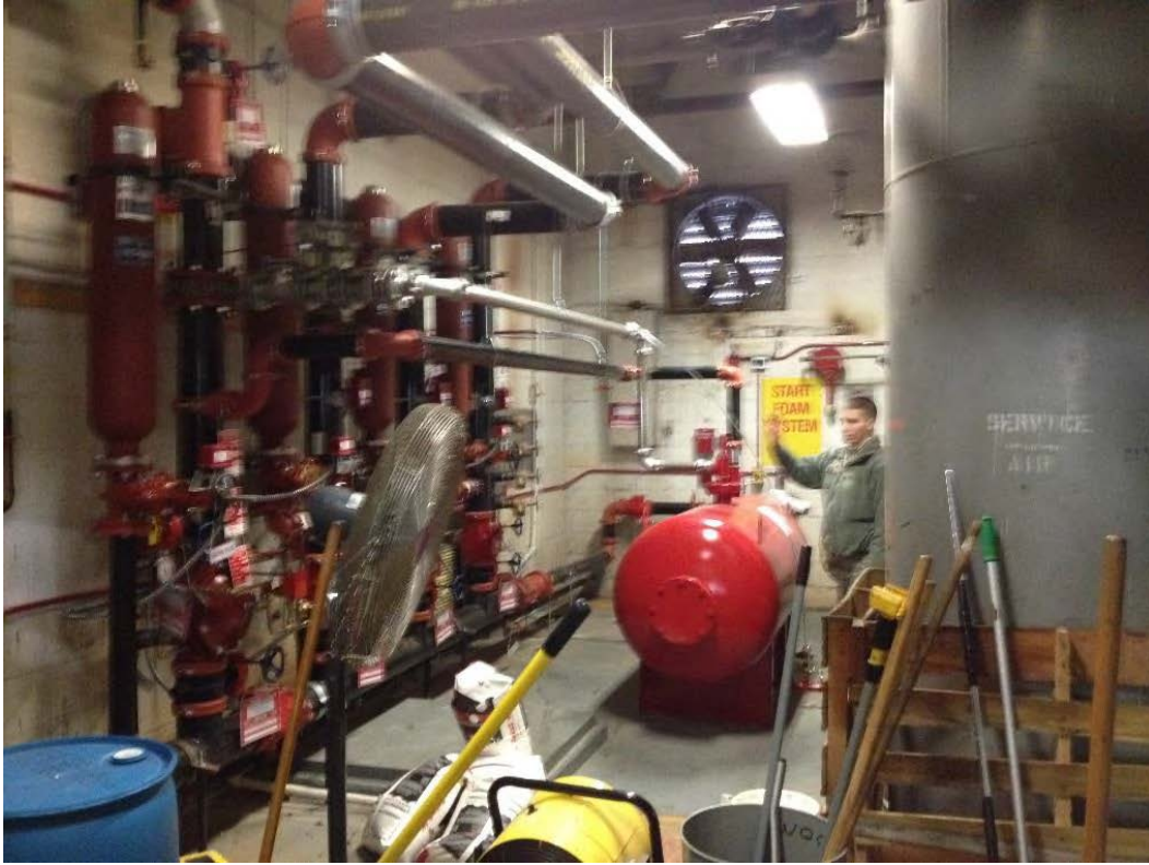
Photo 1: View of Hangar 13 MEC room. HEF system.
