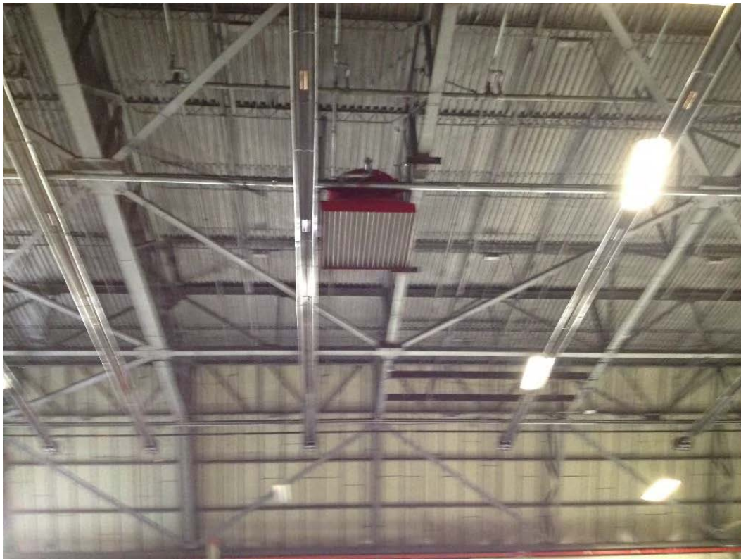
Photo 2: View of fire suppression system in Hangar 12.
