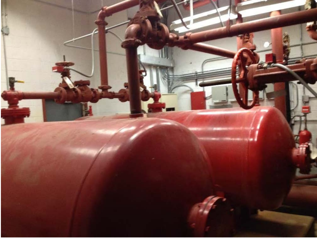
Photo 1: View of Hangar 11 MEC room with twin AFFF tanks.
