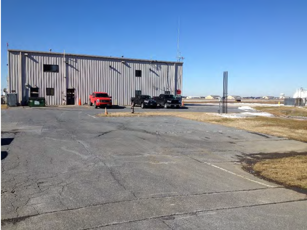
Photo 1: View of Maryland State Police Hangar. BLDG 2487 facing west. OWS captures in the forefront.
