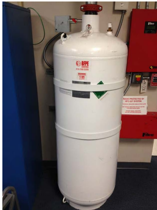
Photo 2: View of BLDG 1539. HFC-227 container.
