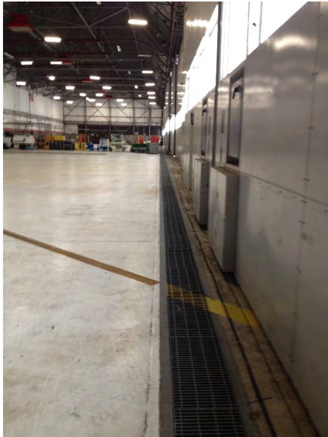
Photo 1: View of fire suppression system in Hangar 14 and trench drain.
