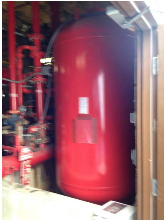
Photo 2: View of BLDG 3302 MEC room with AFFF tank.
