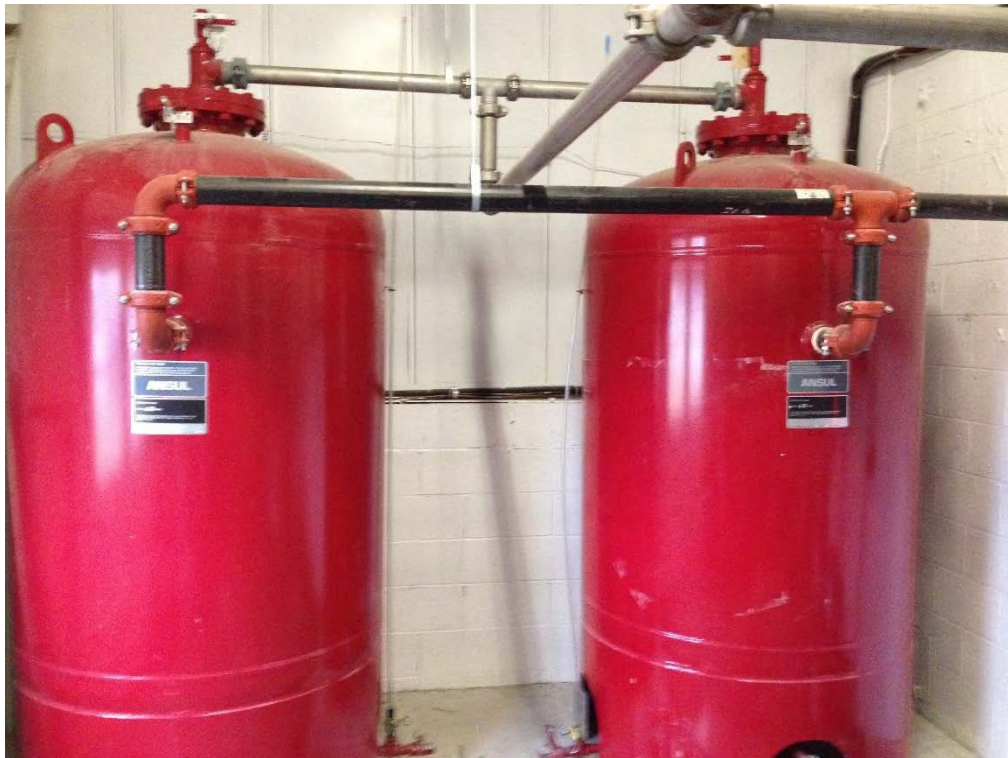
Photo 2: View of Hangar 2 MEC room- HEF.
