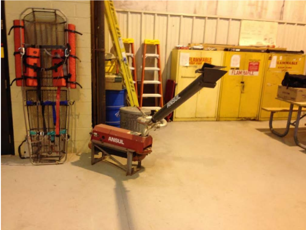
Photo 2: View of Maryland State Police Hangar. BLDG 2487 AFFF floor cannon.
