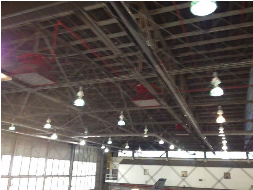
Photo 2: View of fire suppression system in Hangar 16.
