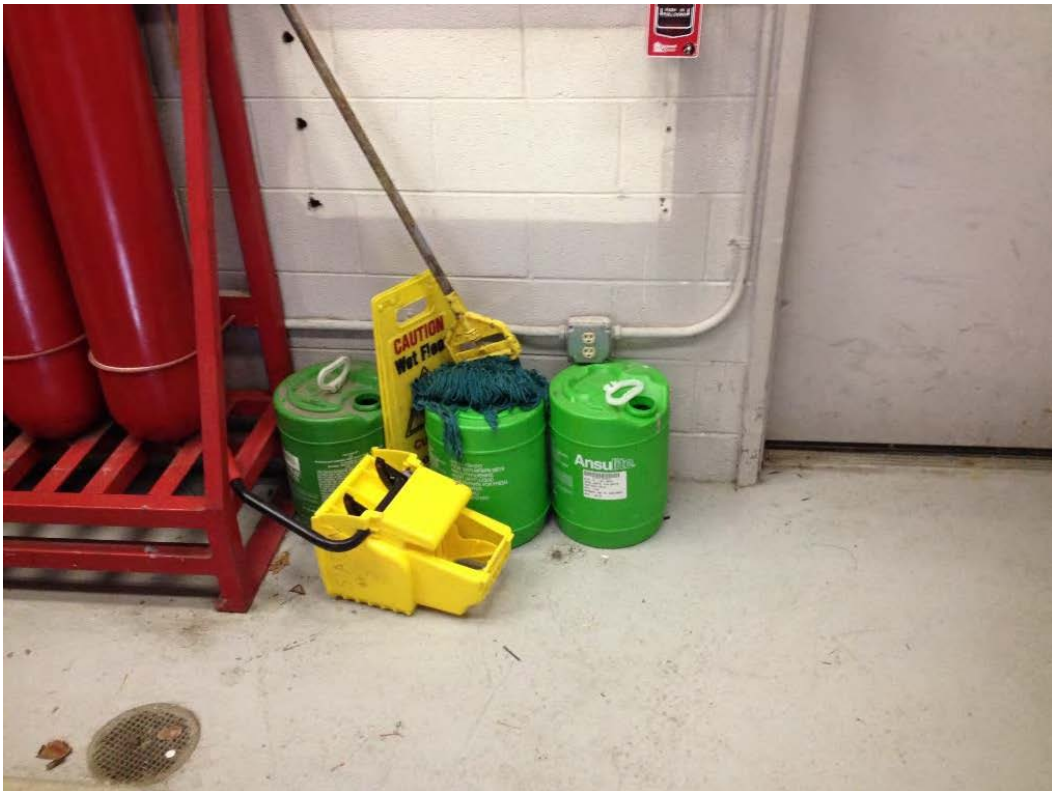
Photo 2: View of Fire Station #2. Empty 5 gallon AFFF buckets.
