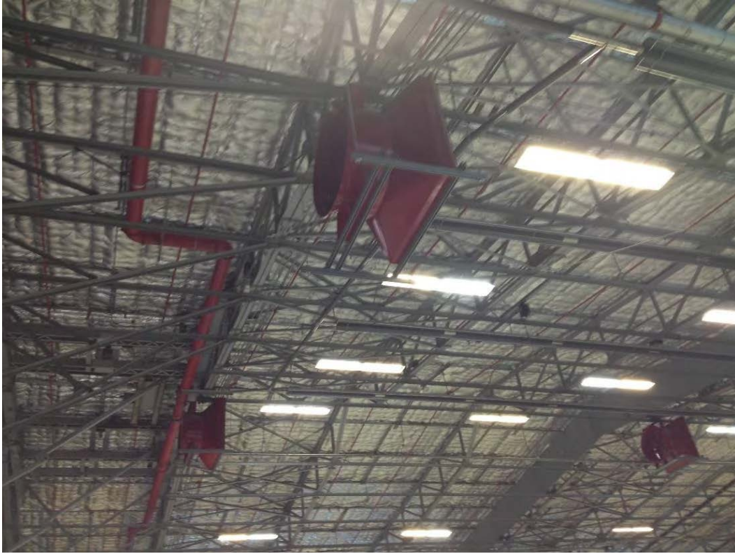
Photo 1: View of fire suppression system in Hangar 5.
