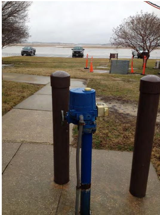
Photo 2: View of Hangar 6 – Automatic isolation valve. Frozen in the open position. Located on east side of Hangar.
